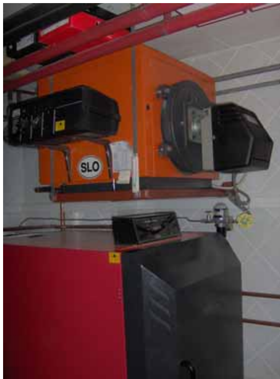
Biomass boiler and oil boiler installed in tandem
