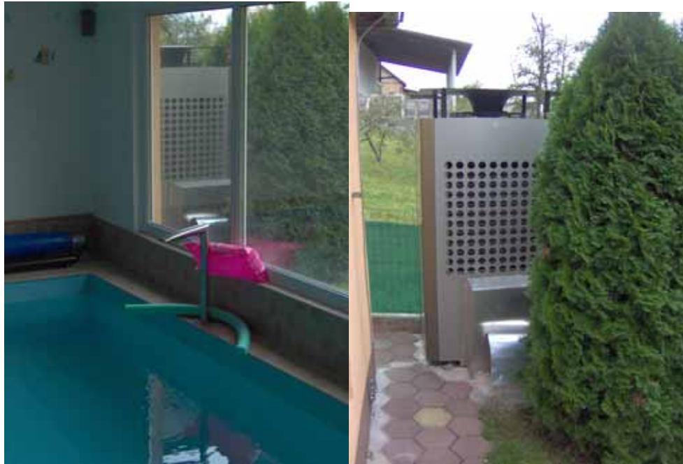
12 KW Air source heat pump and 14 Cu M swimming pool used as heat store
