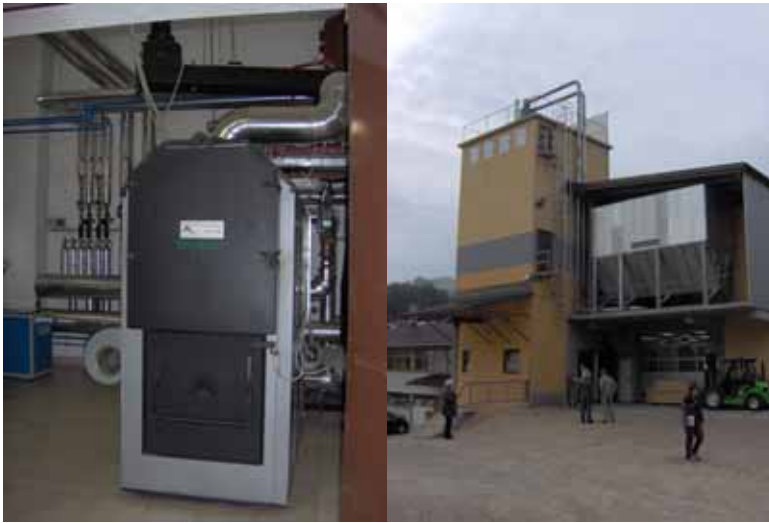
Sawdust waste boiler and sawdust extraction silo
